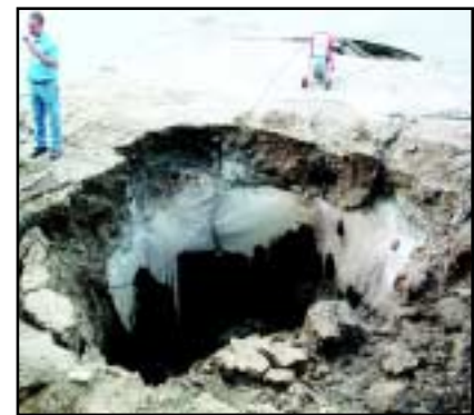
Figure 5-7. Ice-rich permafrost thawing and surface and groundwater intensive flow created this thermokarst pit in a parking lot in Fairbanks, Alaska (photo by V. Romanovsky).
